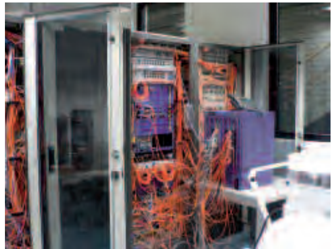
The central network switch at AIP
